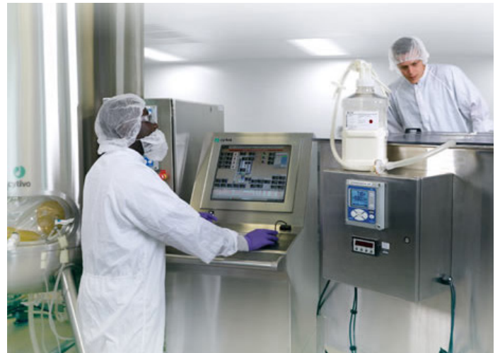
Fig 1. Designed for single unit, multiple units or a fully integrated facility with Rockwell automation's modern DCS platform, PlantPAx®.
